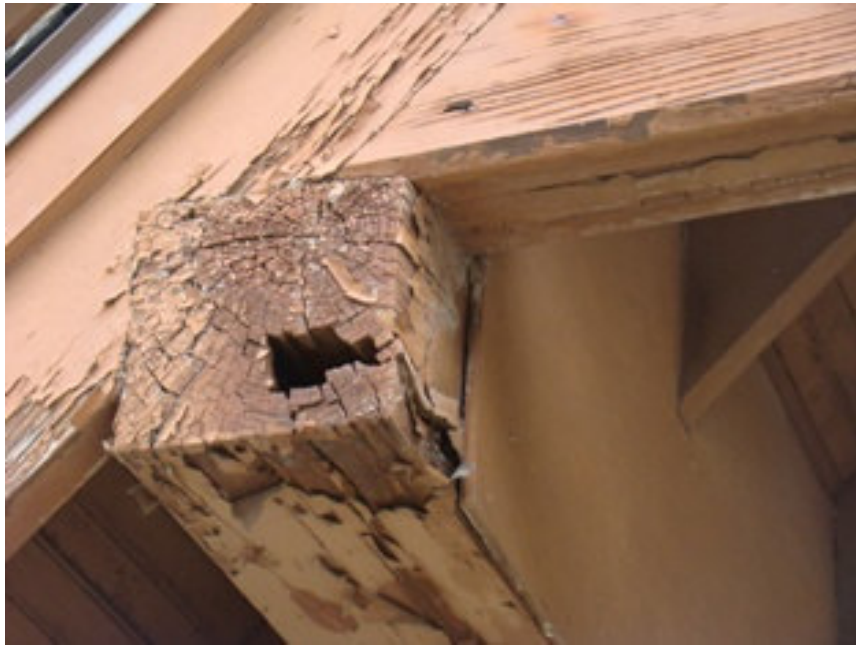
Damage in exterior wooden roof due to rain water
