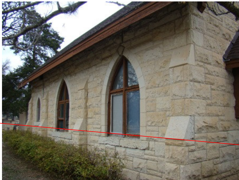
Coping stones in buttresses used as a horizontal Baseline for level comparison
