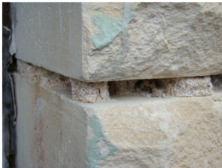
Erosion of original mortar joints due to rain.
