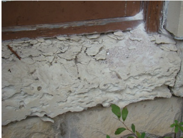
Degradation of window sills.
