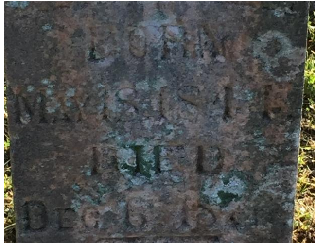
Close-up of D/2 applied, making the growths feasting on the stone even more visible...
